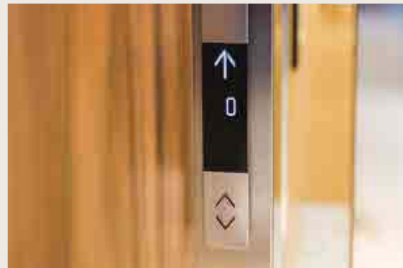
Elevator in each mansion
